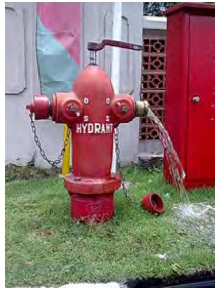
Gambar Hydrant terpasang
