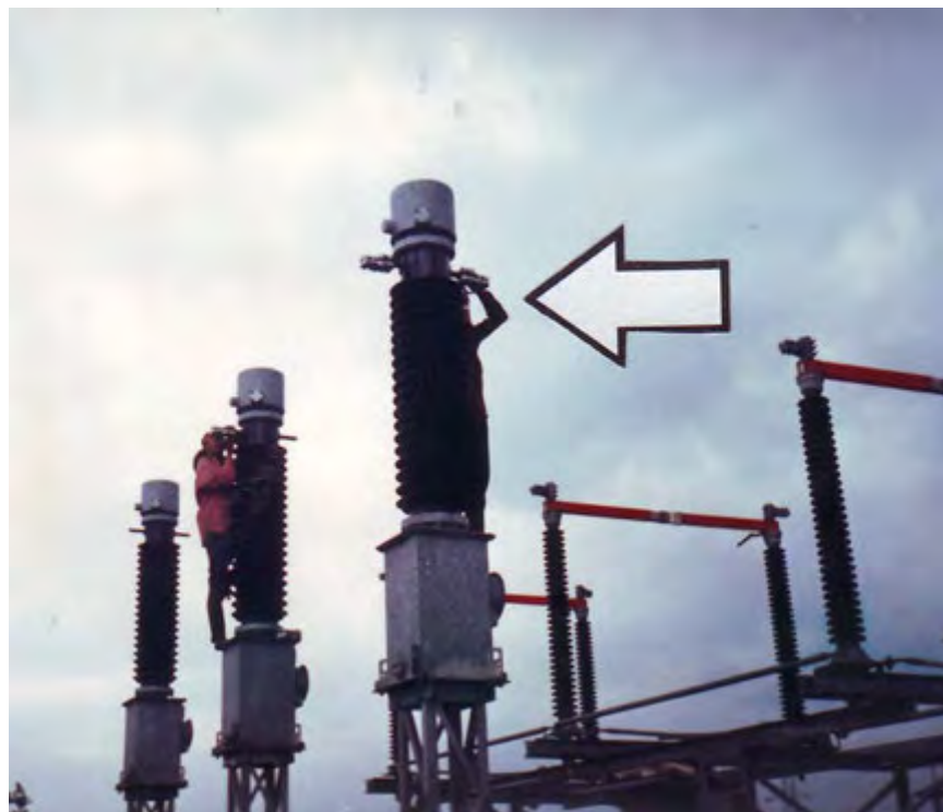
Gambar 3-6. Current Transformer (CT).
