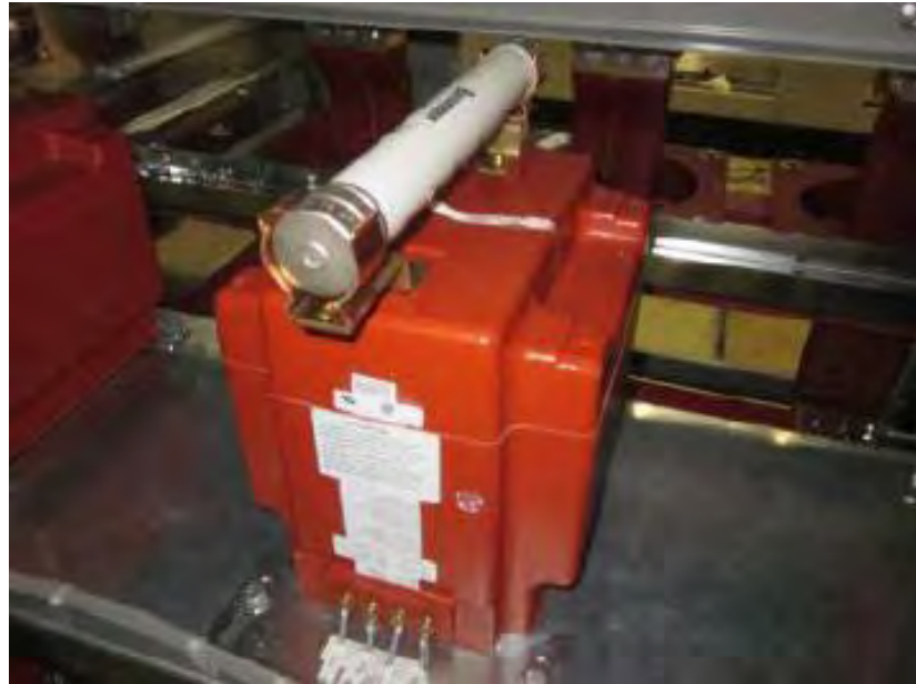
Gambar 3-7. Potential Transformer (PT)
