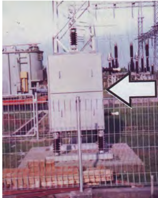
Gambar 3-2. Neutral Grounding Resistance (NGR).
