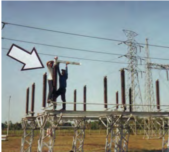
Gambar 3-4. Disconnecting Switch (DS).
