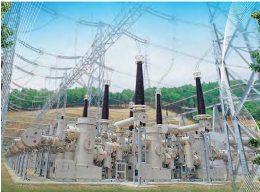
Gambar 2-4. Gas Insulated Substation (GIS).
