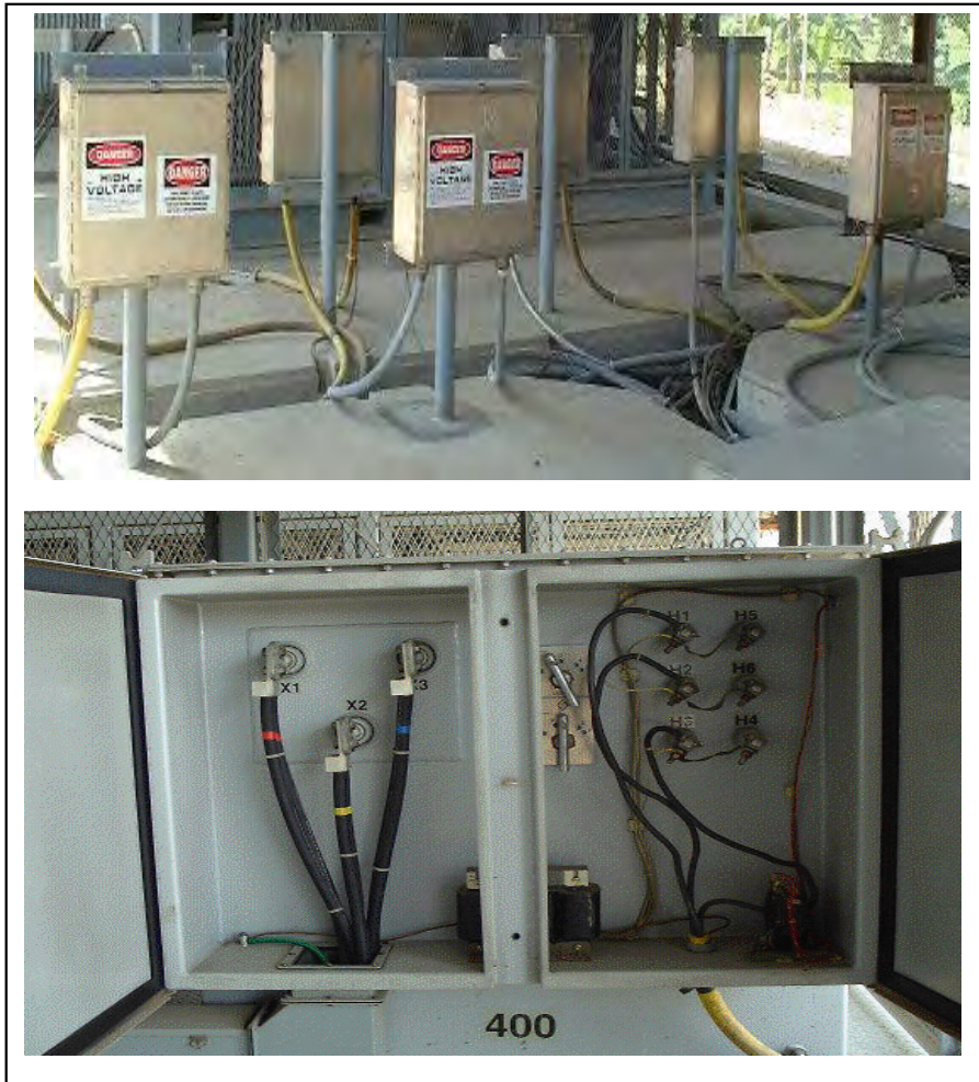
Gambar : Junction Box
